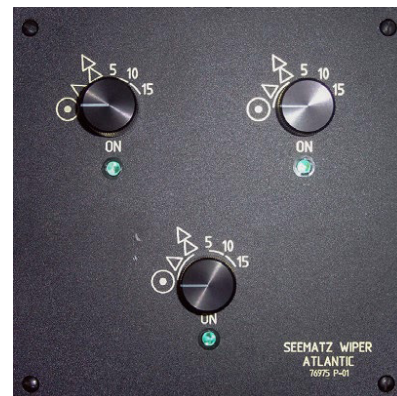
* Example of a control panel, type 'Atlantic'
